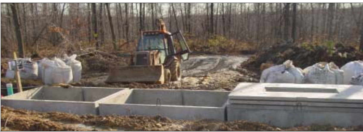
One Co-op RFS III septic system to serve multiple homes - In November 2003, Northwestern Service Corp. installed the first Multi-Residential version of the Co-op RFS III septic system in Venango County. This system works exactly as a single unit - effluent flows from the septic tank into the re-circulating filter tanks then finally passes a UV light before it is discharged. The only difference is that there are three filtering tanks verses two found in a single system. A multi-residential system can serve up to two - four bedroom homes. For more information contact NSC at 1.888.494.8379. ♦
