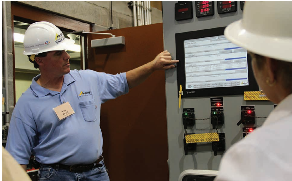
ALLEGHENY OPERATIONS: Eric Reed, lead operations and maintenance technician at the Raystown Hydroelectric Plant, reviews the facility's operating system. Allegheny, formed in 1946 to provide electric cooperatives with a reliable supply of energy at a competitive price, owns and operates the plant in Huntingdon County.
